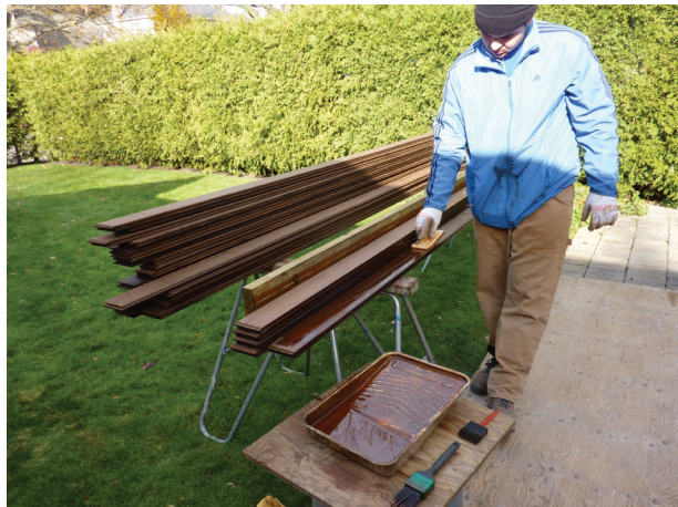
These deck boards are being treated with an oil-based coating. Water-based products can't be used because heat-treated wood doesn't absorb water.
