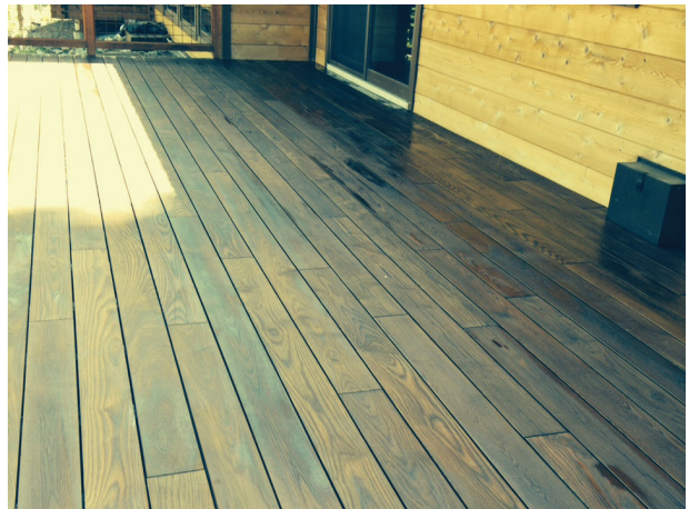
While heat-treated wood quickly turns gray, it can be pressure-washed and re-treated to restore color. This deck was restored after a year in the sun.
